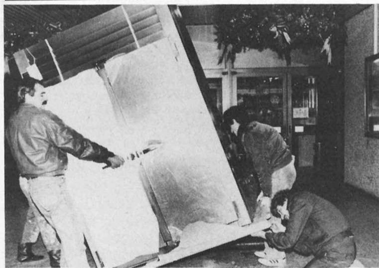
Workers move a refrigeration unit into the new Frank's Franks snack bar.
