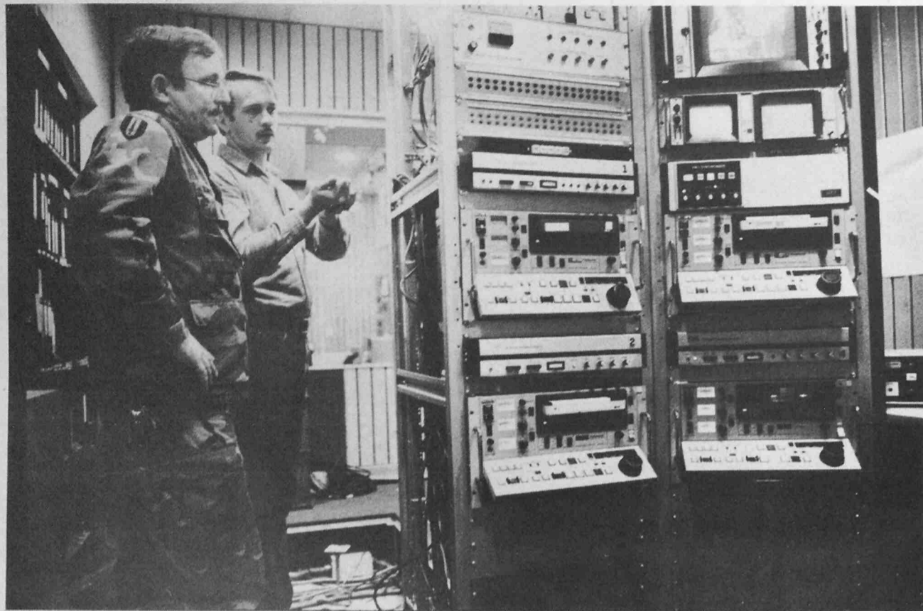
SURVEYING WORK TO BE DONE, SSgt. Allen Schutz, NCOIC of engineering and Chuck Slovak view the heart of AFN-TV's new SATNET operation — the
