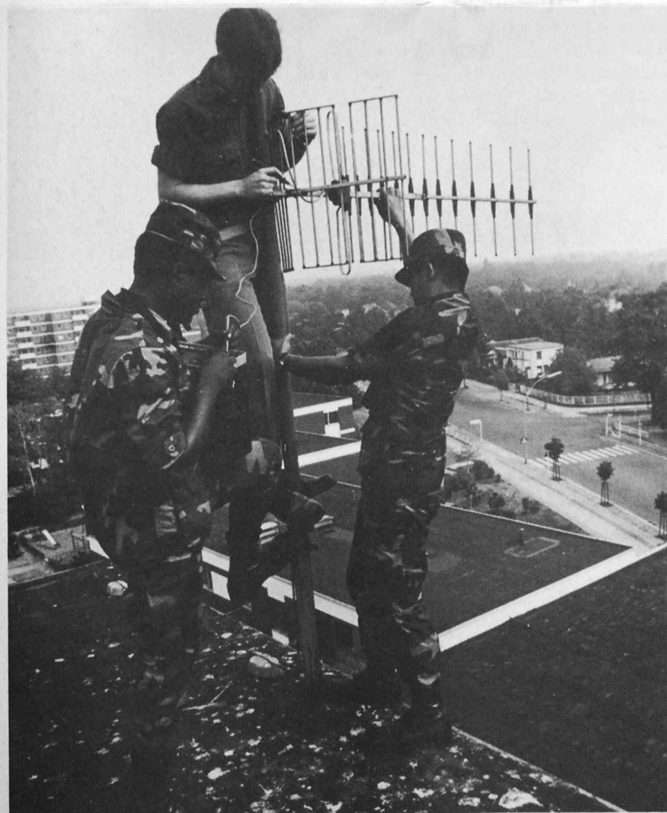
ON THE ROOF —Sp4s Scott Krueger (center), and Cornell Wilkes check the antenna connections on a building in
