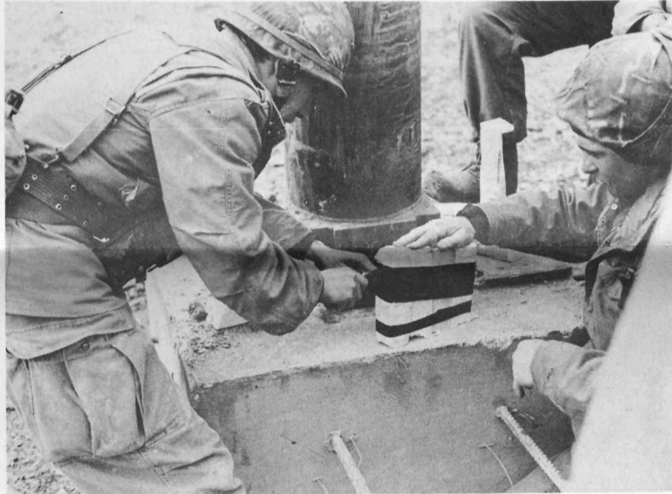
A POWERFUL PACKAGE— Demolition experts from the 42nd Engineer Company, Combat Support Battalion, conduct live-fire exercises while at the Major Training Area at
