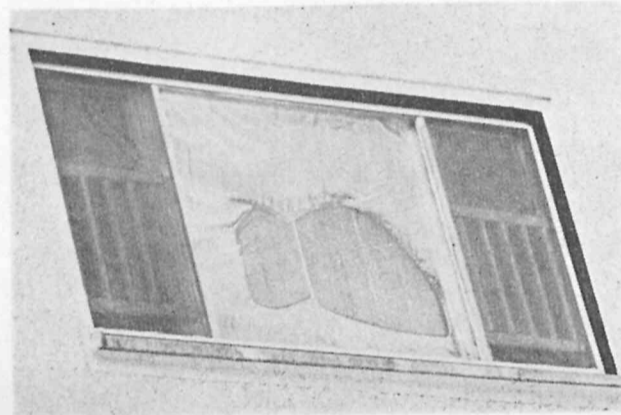
THIS IS WRONG — Someone put plastic on their window in the Berlin Brigade housing area. Moisture collected between the window and the plastic. The wind blew the plastic against the window and it froze there. Since air can not get through the window the mildew problem in this apartment will be aggravated. (Photo by Sandy Redger)
