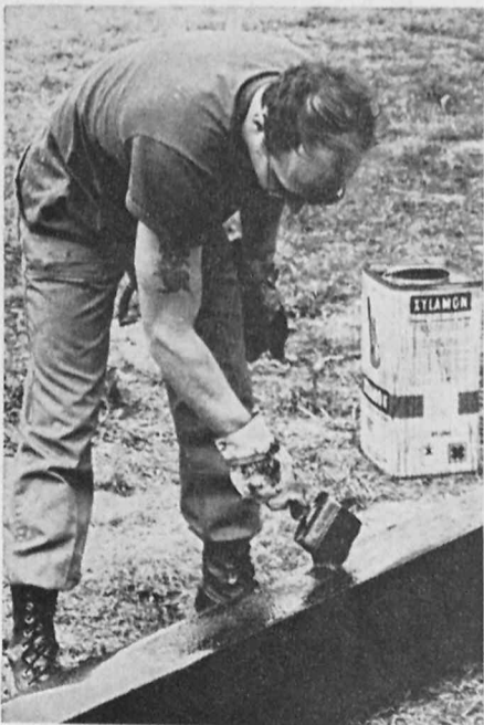
BUILT TO LAST — Sp4 Lee Richmond uses a wood preservative to help keep the new obstacles at Parks Range from deteriorating over the years.
