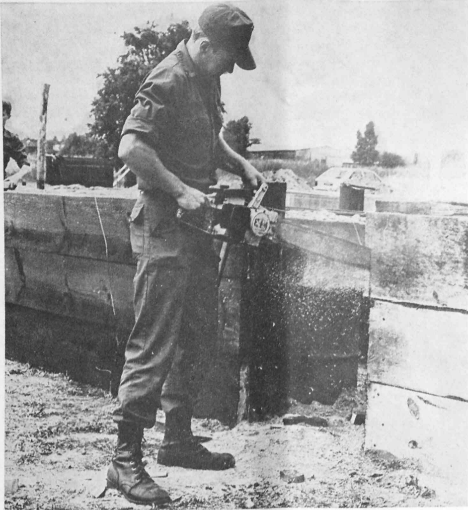
MAKING THE SIDES EVEN — PFC Thomas L. Harbin uses a chainsaw to trim the entrance way of the "Barrel Maze," one of the new obstacles that
