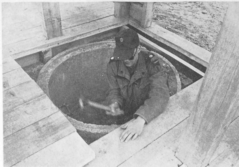
TAP, TAP, TAP — Sgt. Kip T. Berentson, 2nd Platoon, 42nd Engineer Company, Combat Support Battalion, hammers in the last nail. This
