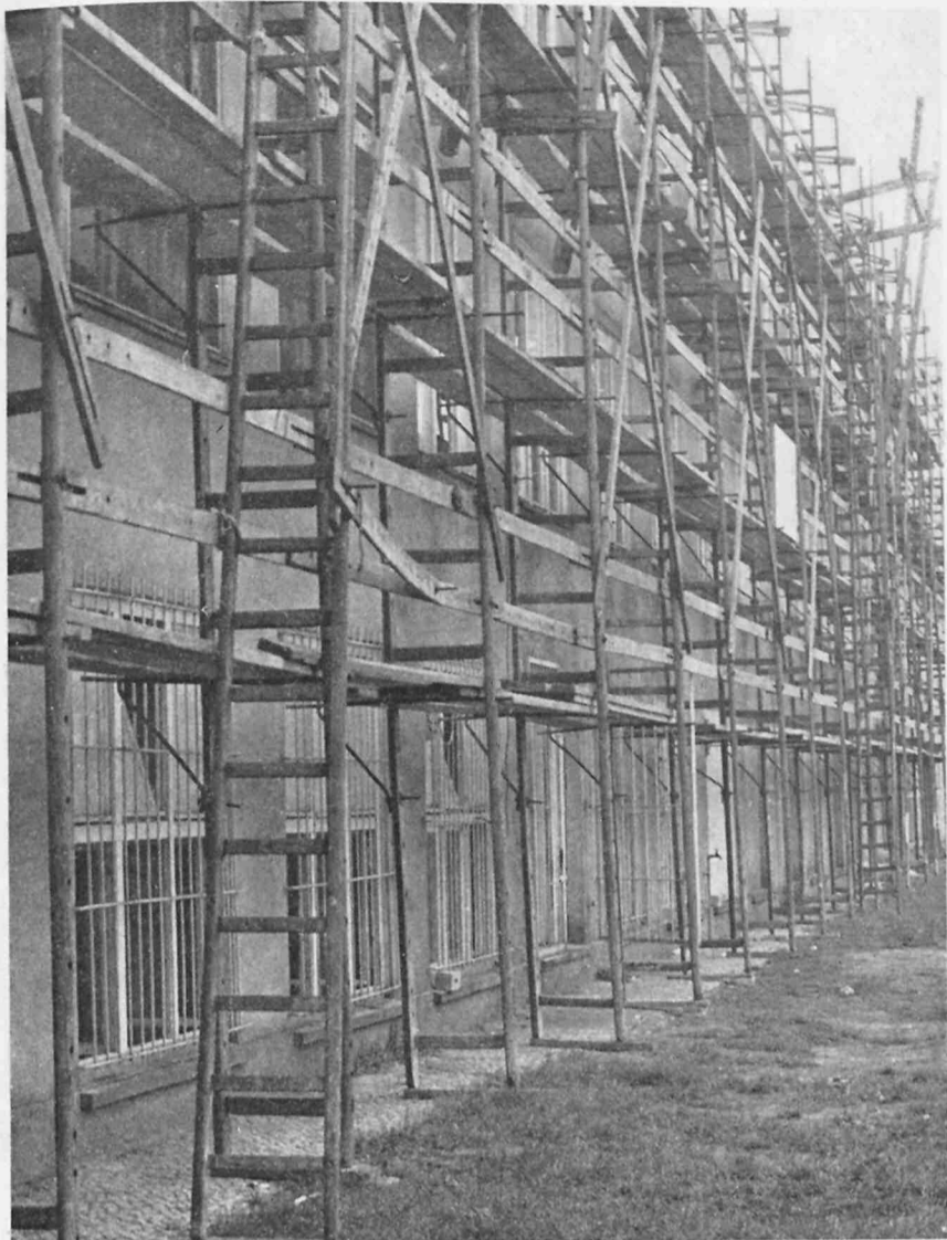
NEW LOOK — Work continues on the billets of the 3rd Battalion, 6th Infantry at McNair Barracks as the exterior of the building gets a complete facelift. Work will also be done to modernize the interior of the quarters. (Photo by SP5 Dan Fredrickson)
