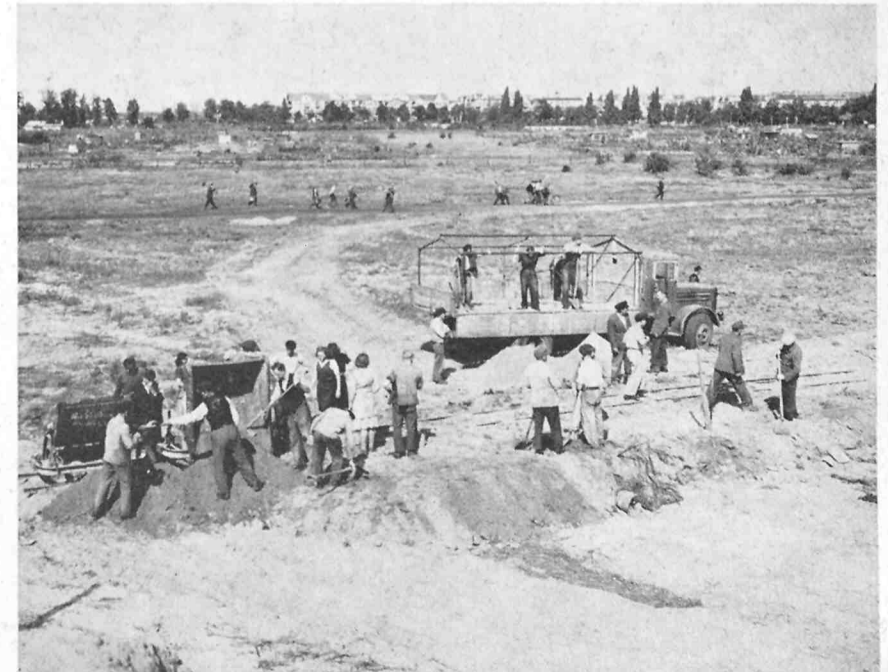
WORKING ON THE RAILROAD — New runways were added to Tempelhof and Gatow Airports but to relieve the load it was necessary to build a new airport. Tegel Airfield, in the French Sector of Berlin, was opened for Airlift operations December 7, 1948 and within a few short weeks it became a major terminal.
