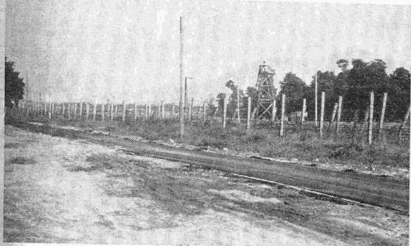
JOINT PROJECT COMPLETED —Above is a portion of a new road constructed by the 42d Engineer Company and the city of Berlin. This morning the road was to be officially opened for border patrol vehicles.
